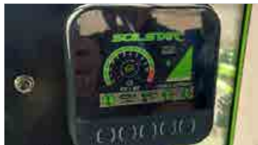
ELECTRIC CONTROL MONITOR
